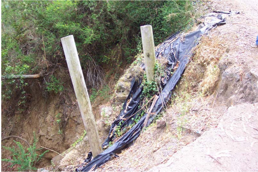
Figure 104: Ineffective erosion control structures. Tarps have washed downslope over the sandbags supporting the trail in just one rainy season.
